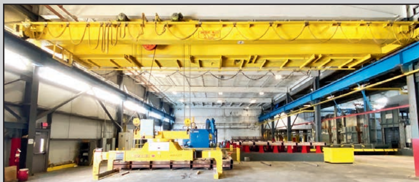
SAMPLE BRIDGE CRANE
