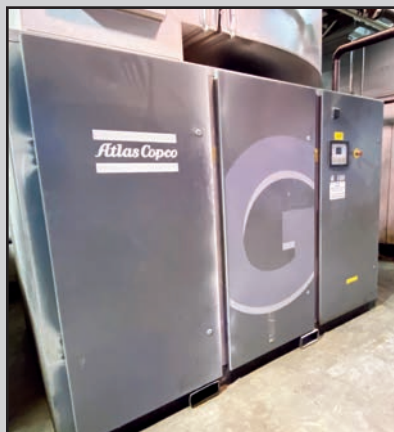
(2) ATLAS COPCO 200 HP ROTARY SCREW AIR COMPRESSORS
